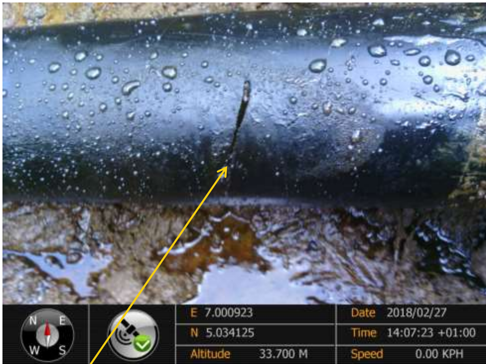
Close-up: Hacksaw cut on 4" Otamiri Well5LS Flowline at Abara. Picture was taken during Joint Investigation of 27 th February 2018.
