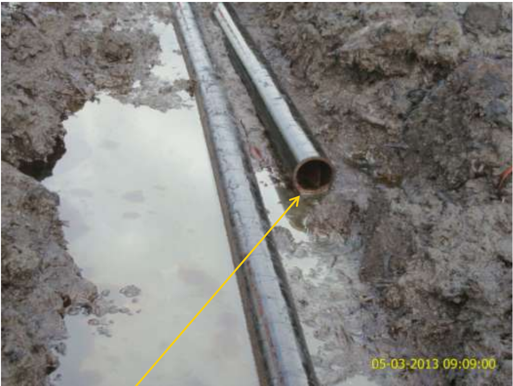
Close up: Missing flowline section on 4" Awoba North West Well L & S flowlines at Boro. Picture was taken during Joint Investigation of 5 th March 2013.
