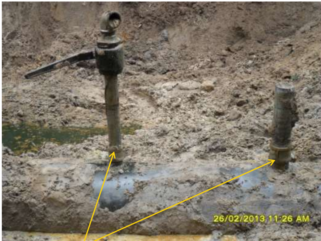
Close up: Illegal fittings on 18" Assa-Rumuekpe pipeline at Elele-Alimini. Picture was taken during Joint Investigation of 26 th February 2013.
