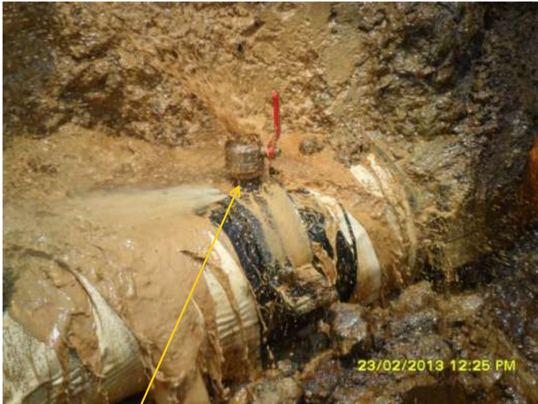
Close up: Illegal fitting on 12" Imo River – Ogale pipeline at Uzuaku. Picture was taken during Joint Investigation of 23 rd February 2013.
