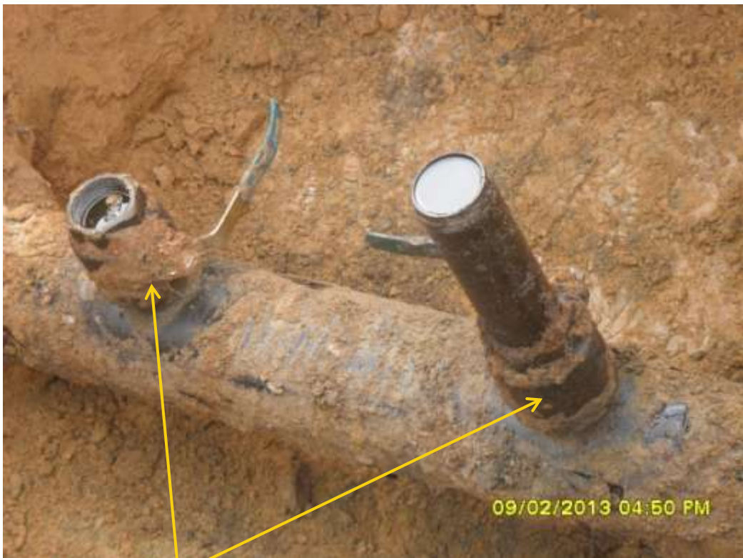
Close up: Illegal fittings on 8" Umuechem-Nkpoku pipeline at Omunwei. Picture was taken during Joint Investigation of 9 th February 2013.
