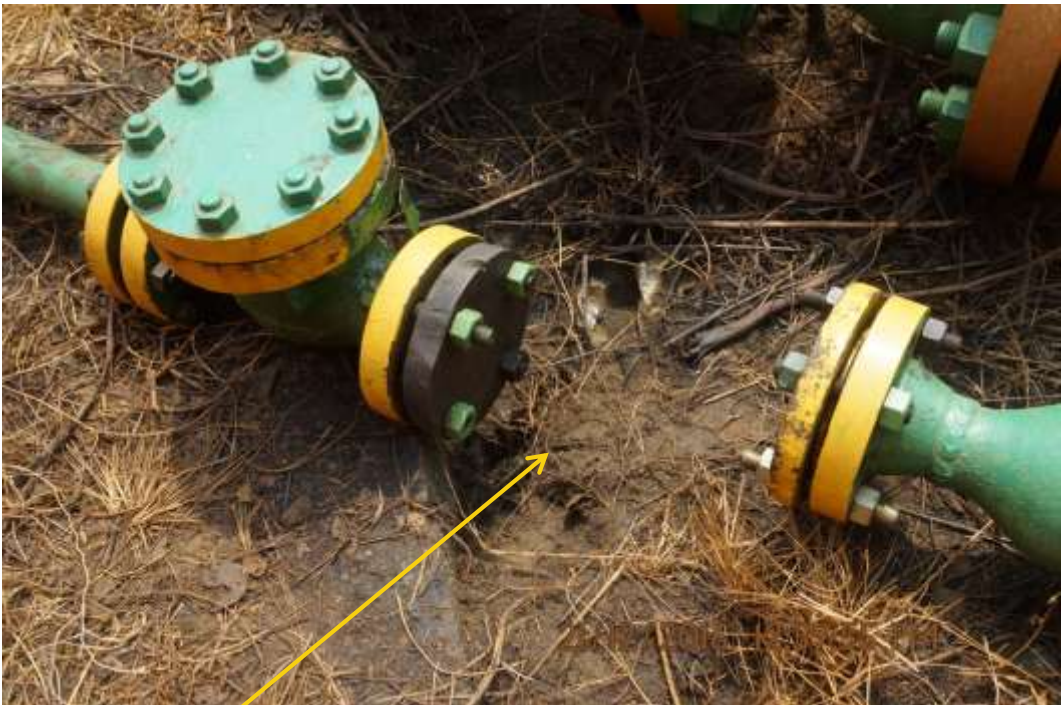
Close-up: Position of missing valve on 2" Yokri Well127T Gas Lift Line at Yokri. Picture was taken during Joint Investigation of 21 st December 2016.
