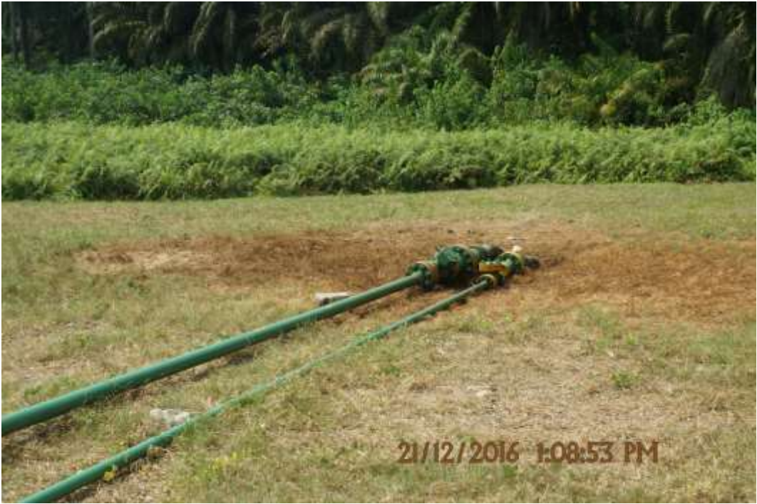
Overview: Location of spill around 2" Yokri Well127T Gas Lift Line at Yokri. Picture was taken during Joint Investigation of 21 st December 2016.
