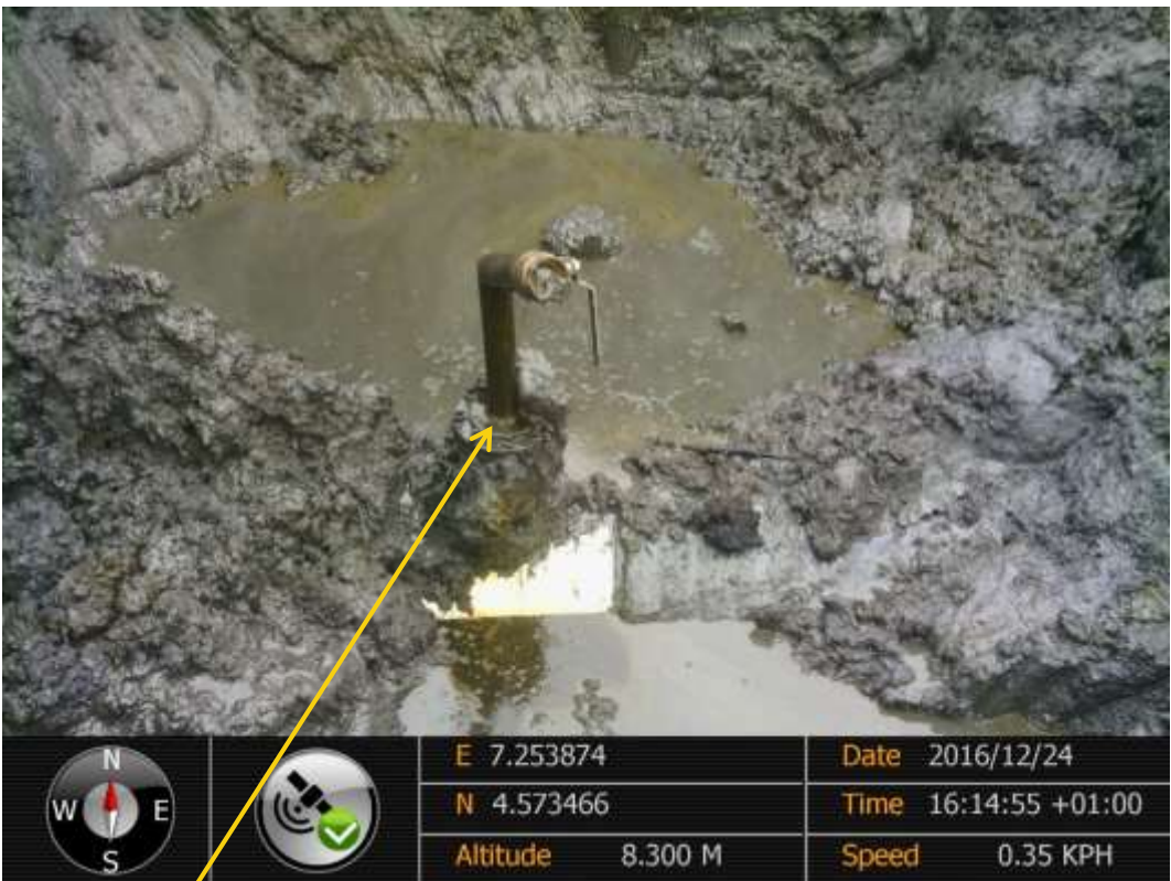
Close-up: Illegal fitting on 28" Bomu-Bonny Pipeline at Bodocity. Picture was taken during Joint Investigation of 24 th December 2016.
