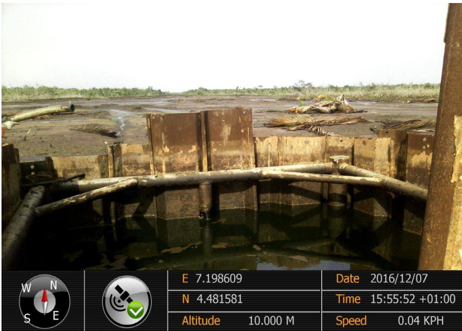
Overview: Part of spill impact on 28" Bomu-Bonny Pipeline at Okolomabio-Oloma. Picture was taken during Joint Investigation of 7 th December 2016.
