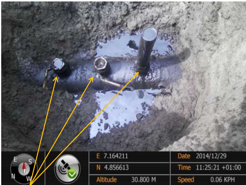
Close-up: Illegal fittings on 12" Imo River – Ogale Pipeline at KomKom. Picture was taken during Joint Investigation of 29 th December 2014.
