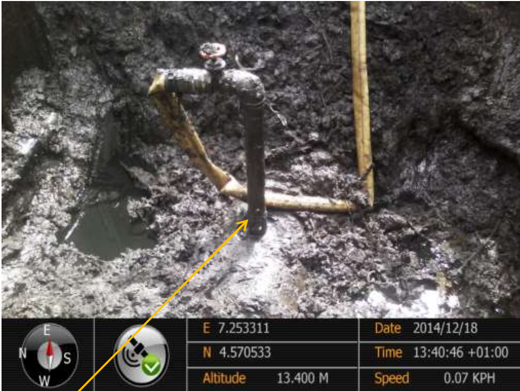
Close-up: Illegal fitting on 28" Bomu-Bonny Pipeline at Bodo City. Picture was taken during Joint Investigation of 18 th December 2014.
