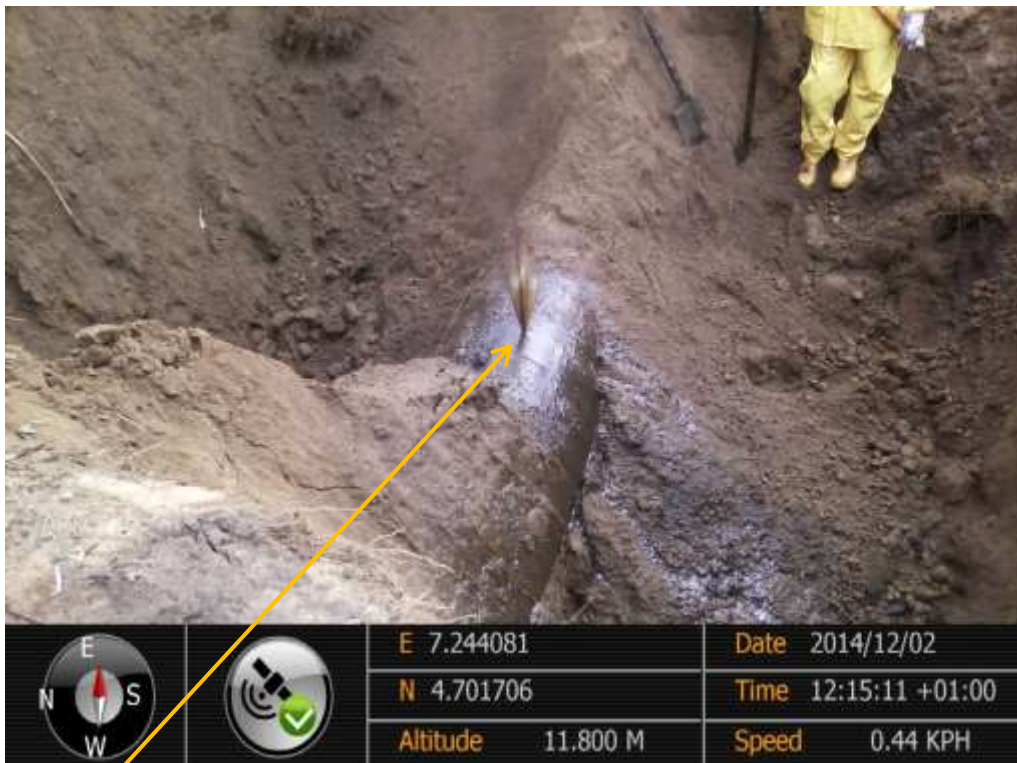
Close-up: Spill due to drilled hole on 28" Nkpoku-Bomu Pipeline at Gio. Picture was taken during Joint Investigation of 2 nd December 2014.
