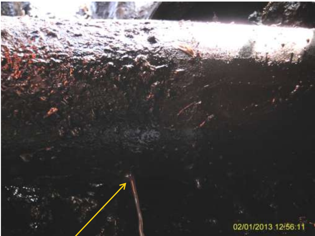
Close up: Spill due to corrosion on Cawthorne Channel Well41S flowline at Elemama. Picture was taken during Joint Investigation of 2 nd January 2013.
