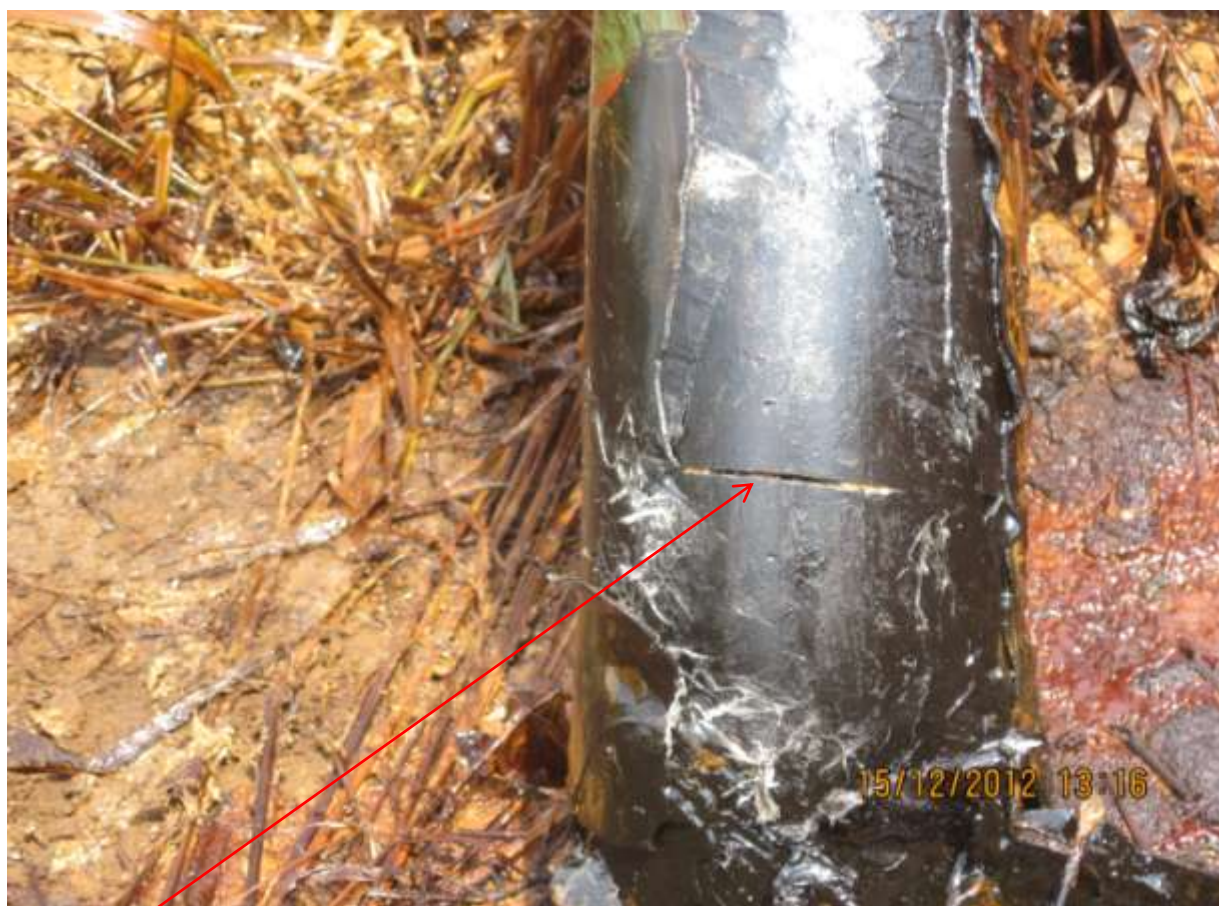
Close-up: Hacksaw cut on Umuechem Well 12L flowline at Umuechem. Picture was taken during Joint Investigation of 15 th Dec. 2012.
