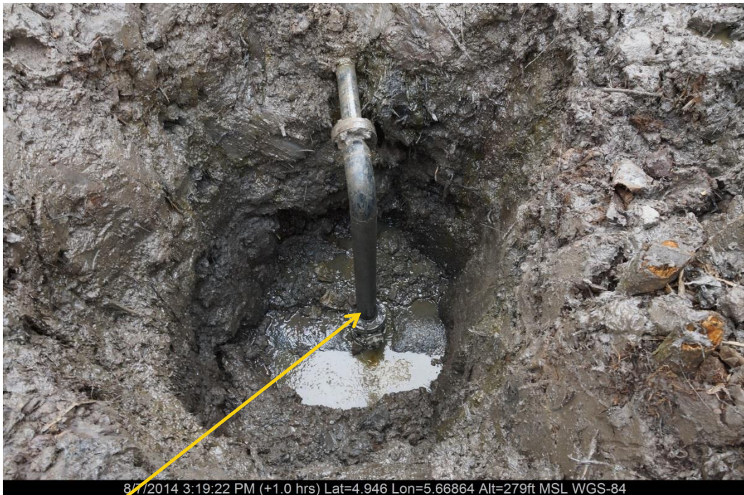
Close-up: Illegal fitting on 20" Opukushi-Brass Creek Pipeline at Peretourgbene. Picture was taken during Joint Investigation of 7 th August 2014.
