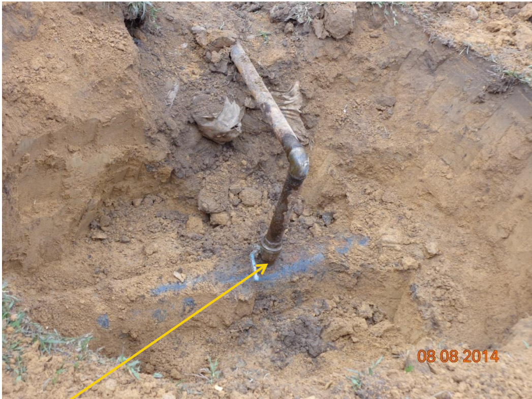
Close-up: Illegal fitting on 8" Obigbo North - New Eelenwo at Umukolobe . Picture was taken during Joint Investigation of 8 th August 2014.
