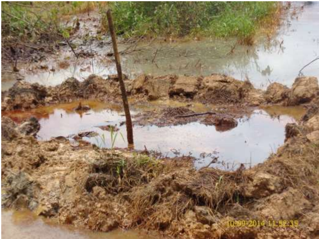
Overview: Part of spill impact on 10" Diebu Creek – Nun River Pipeline Right of Way at Ekowe. Picture was taken during Joint Investigation of 10 th September 2014.
