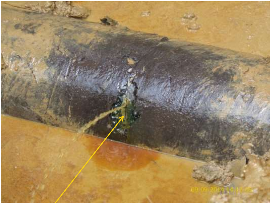
Close-up: Hacksaw cut on 10" Diebu Creek – Nun River Pipeline at Ekowe. Picture was taken during Joint Investigation of 9 th September 2014.
