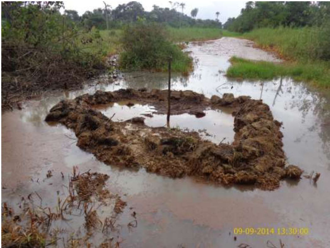
Overview: Spill location on 10" Diebu Creek – Nun River Pipeline Right of Way at Ekowe. Picture was taken during Joint Investigation of 9 th September 2014.
