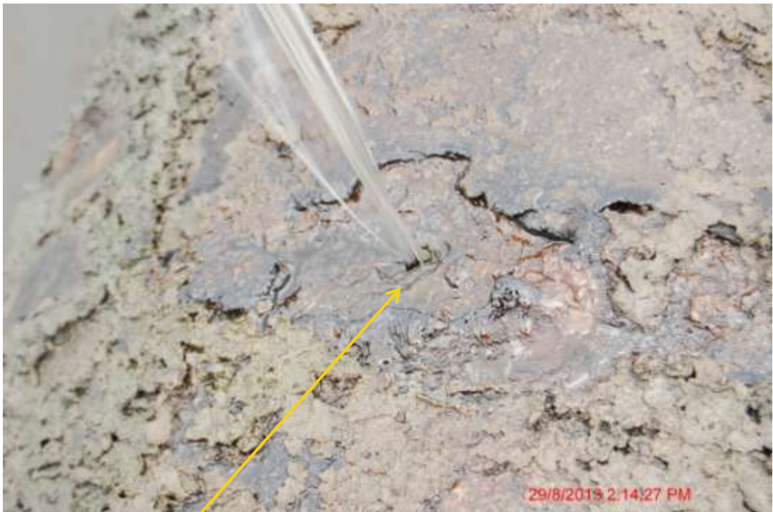
Close up: Hole due to corrosion on 24" Alakiri-Bonny pipeline at Ilomaturu. Picture was taken during Joint Investigation of 29 th August 2013.
