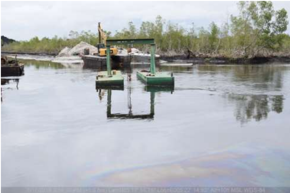
Overview: Part of spill impact on 24" Trans-Ramos Pipeline Right of Way at Odimodi. Picture was taken during Joint Investigation of 17 th July 2018.
