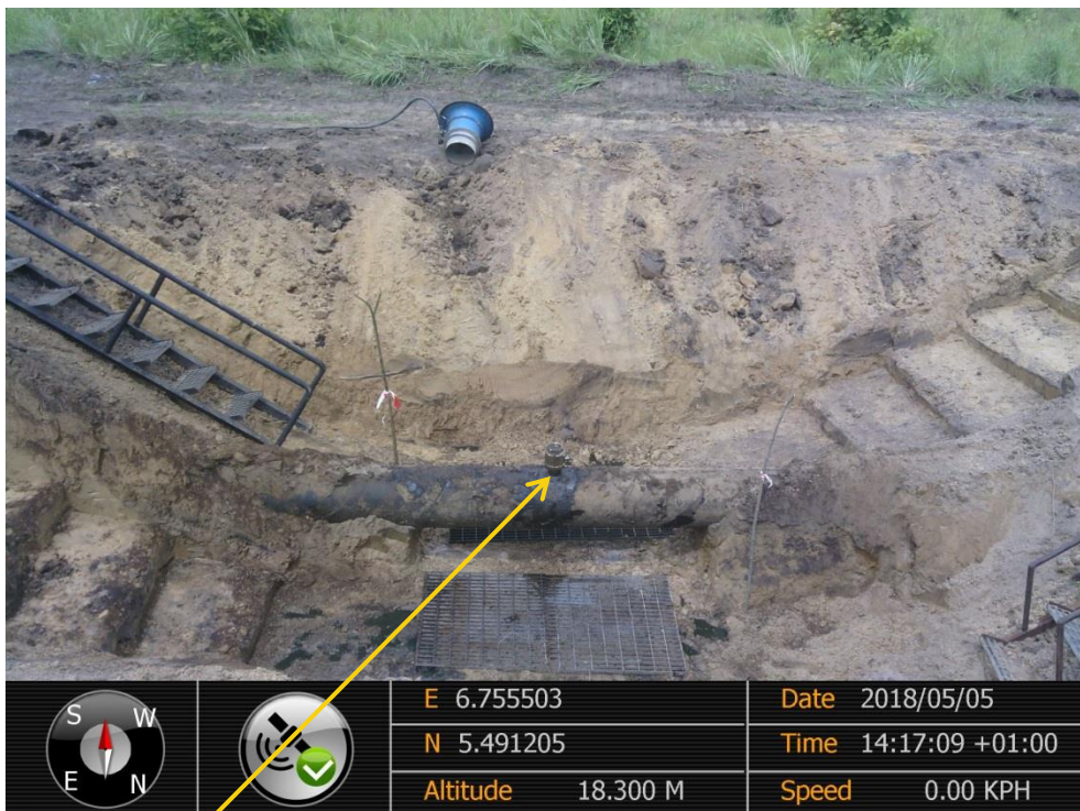
Close-up: Illegal Fitting on 16" Egbema-Assa Pipeline at Ekugba. Picture was taken during Joint Investigation of 5 th May 2018.
