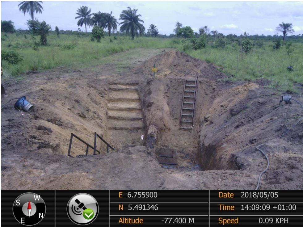
Overview: Part of spill impact on 16" Egbema-Assa Pipeline at Ekugba. Picture was taken during Joint Investigation of 5 th May 2018.
