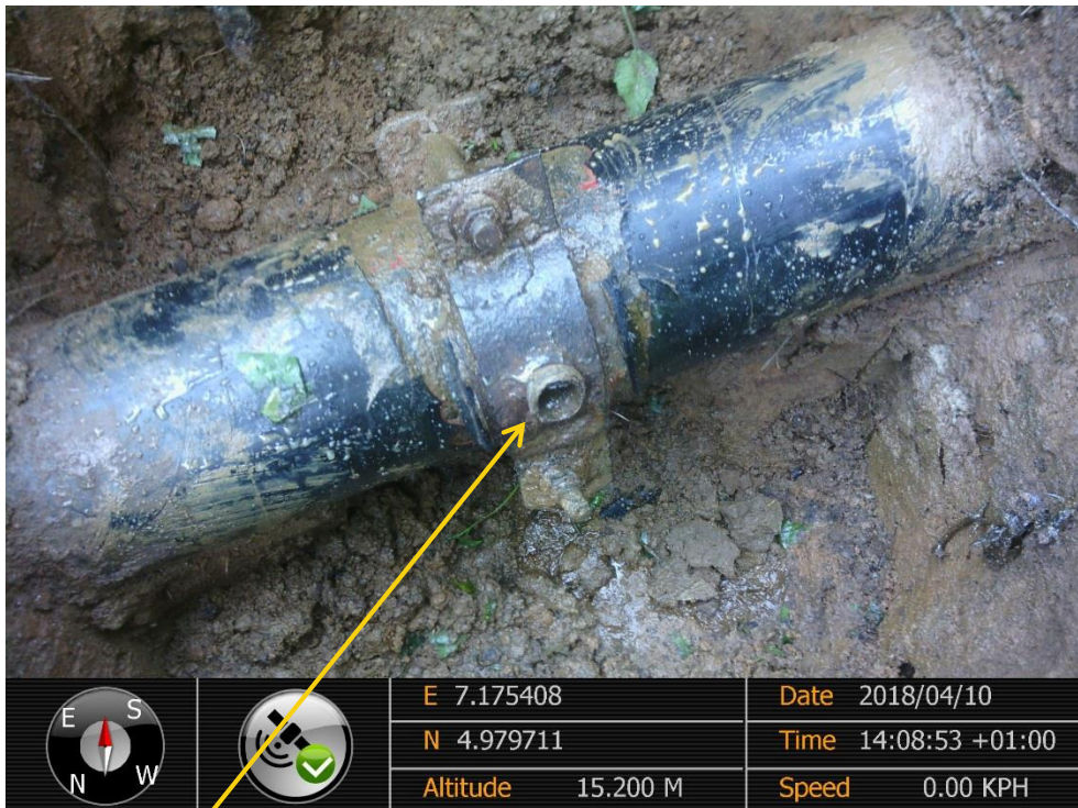
Close-up: Failed Half Inch Nipple on Imo River Well 31S 6" Flowline at Owaza. Picture was taken during Joint Investigation of 10 th April 2018.
