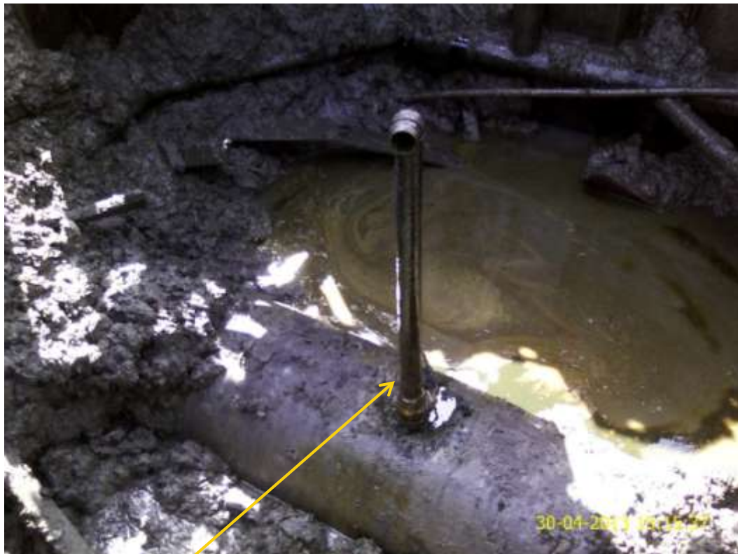
Close up: Illegal fitting on 30" NembeCreek pipeline at Bille. Picture was taken during Joint Investigation of 30 th April 2013.
