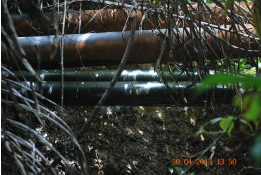
Overview: Part of spill impact on 6" Adibawa North East bulkline right of way at Biseni. Picture was taken during Joint Investigation of 30 th April 2013.
