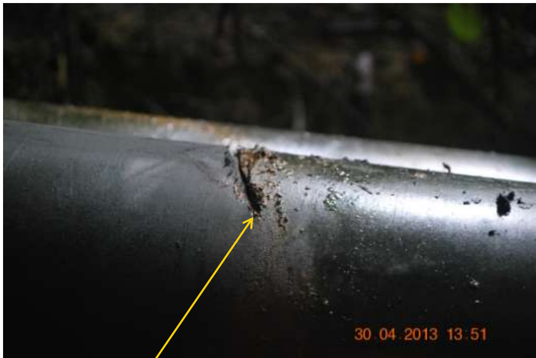
Close up: Hacksaw cut on 6" Adibawa North East bulkline at Biseni. Picture was taken during Joint Investigation of 30 th April 2013.
