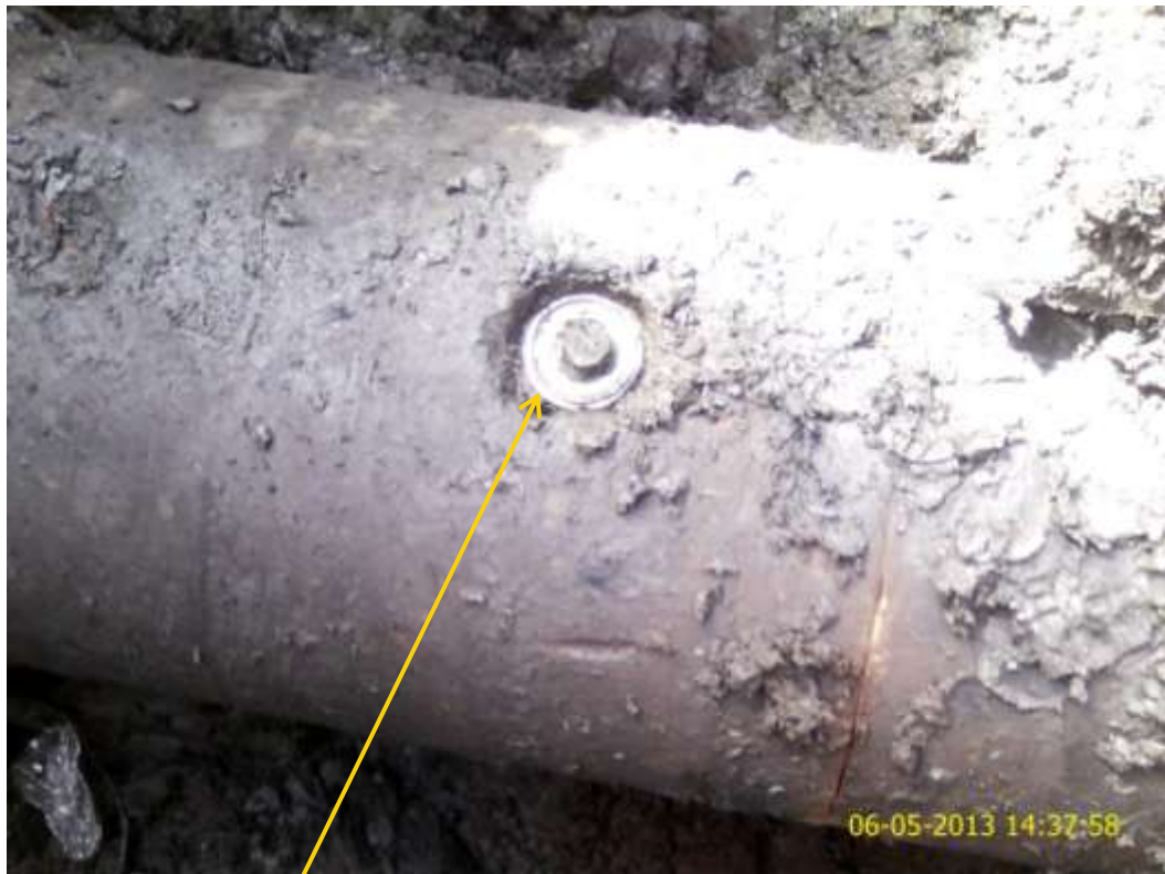
Close up: Illegal fitting on 30" NembeCreek pipeline at Bille. Picture was taken during Joint Investigation of 6 th May 2013.
