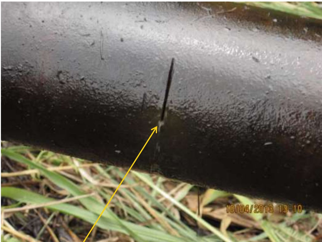
Close up: Hacksaw cut on Adibawa Well8S flowline at Edagberi. Picture was taken during Joint Investigation of 10 th April 2013.
