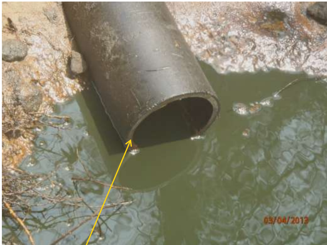
Close up: Cut section on Imo River 4" Well64L flowline at Igiriukwu. Picture was taken during Joint Investigation of 3 rd April 2013.
