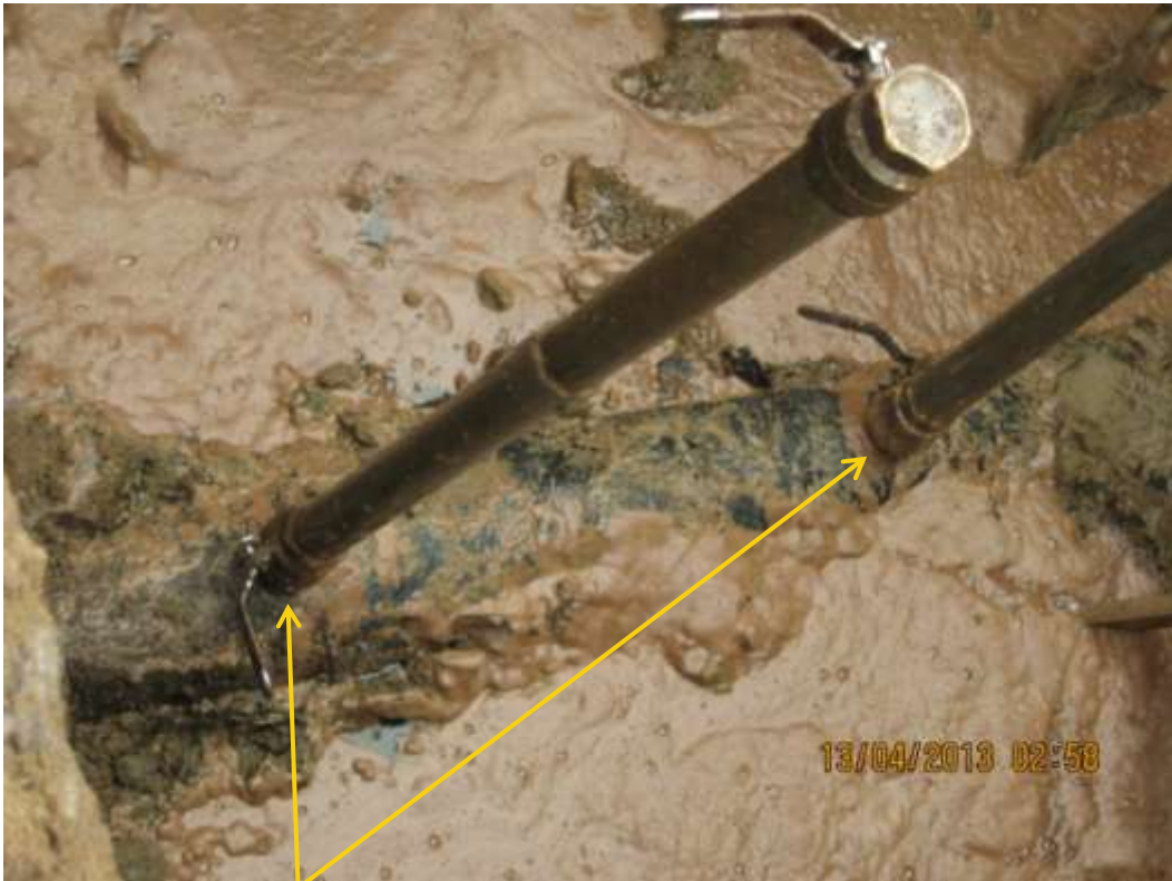
Close up: Illegal fittings on 8" Nkali pipeline at Umuedeokwara. Picture was taken during Joint Investigation of 13 th April 2013.
