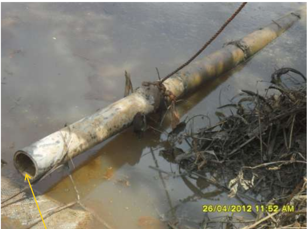
Close up: Cut section on KoloCreek Well3T flowline at Otusega. Picture was taken during Joint Investigation of 26 th April 2012.
