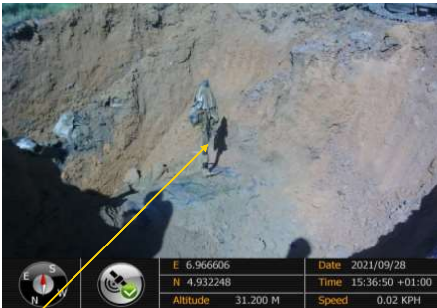
Close-up: 2inch ball valve installed at 12 o'clock position on 36" Rumuekpe Nkpoku Pipeline at Mbodo-Aluu. Picture was taken during Joint Investigation of 28 th September 2021.
