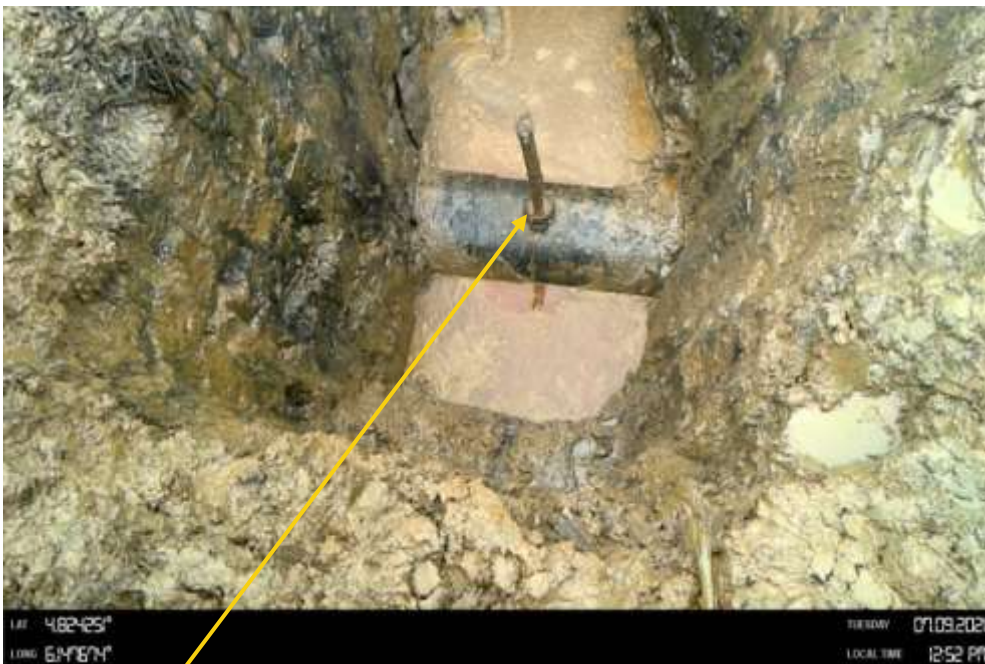
Close-up: Plugged 3inch nipple installed at 12 o'clock position on 16" Nun River Kolocreek Pipeline at Aguobiri. Picture was taken during Joint Investigation of 7 th September 2021.
