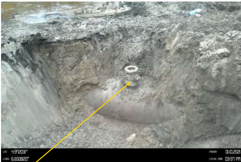
Close-up: 4" ball valve installed at 12 o'clock position on 20" Kolocreek – Rumuekpe Pipeline at Okoma . Picture was taken during Joint Investigation of 1 st October 2021.
