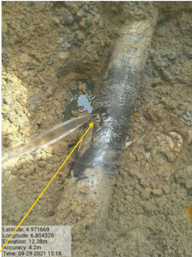
Close-up: Hacksaw cut at 9-11 o'clock position on 4" Obele Ibaa Delivery line at Ibaa. Picture was taken during Joint Investigation of 29 th September 2021.
