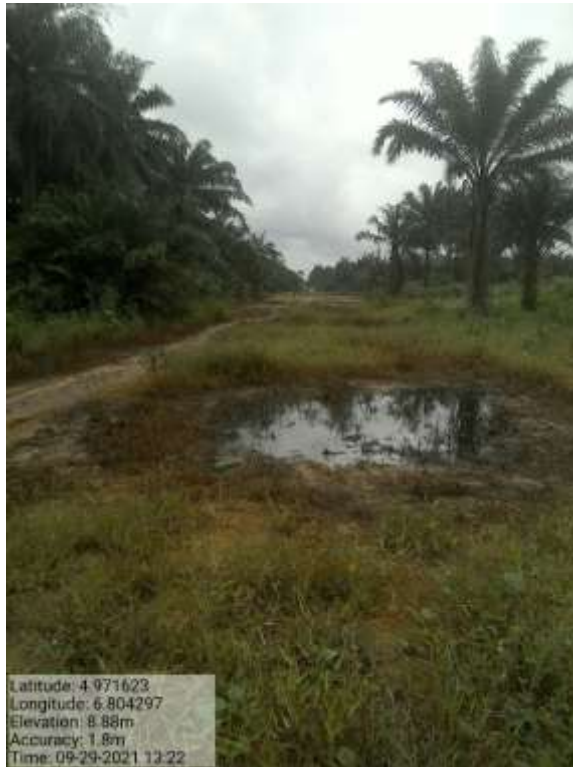
Overview: Part of spill impact on 4" Obele Ibaa Delivery line at Ibaa. Picture was taken during Joint Investigation of 29 th September 2021.
