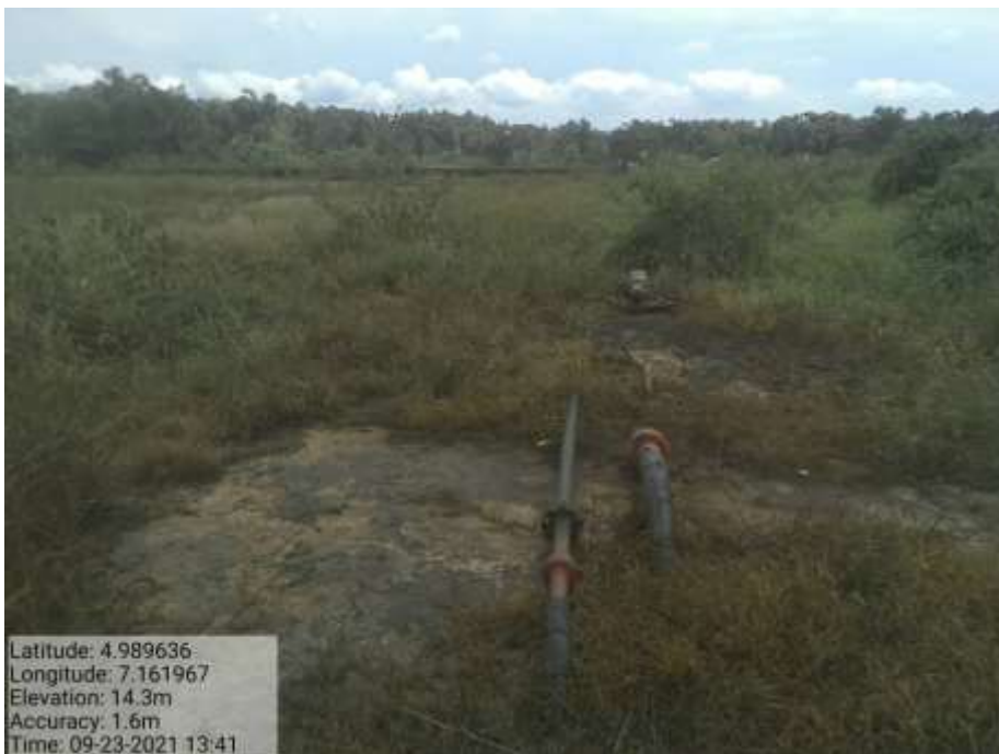
Close-up: Missing Flowline on 4" ImoRiver well 58T flowline at Odagwa. Picture was taken during Joint Investigation of 23 rd September 2021.
