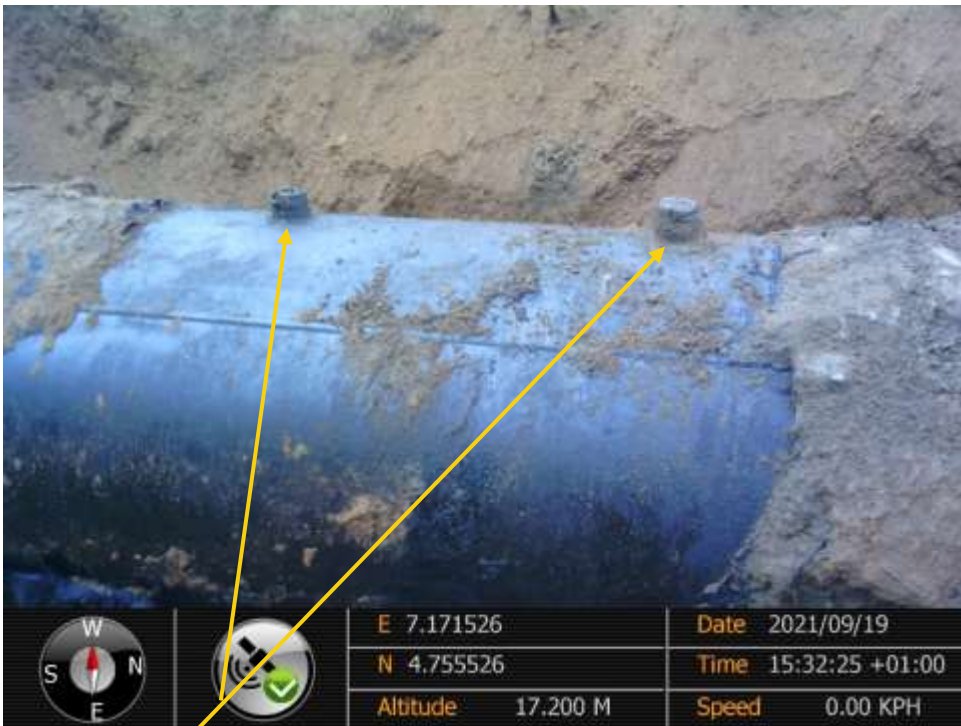
Close-up: 2nos of 2inch nipple installed at 12 o'clock position on 28" Nkpoku Bomu Pipeline at Eteo. Picture was taken during Joint Investigation of 19 th September 2021.
