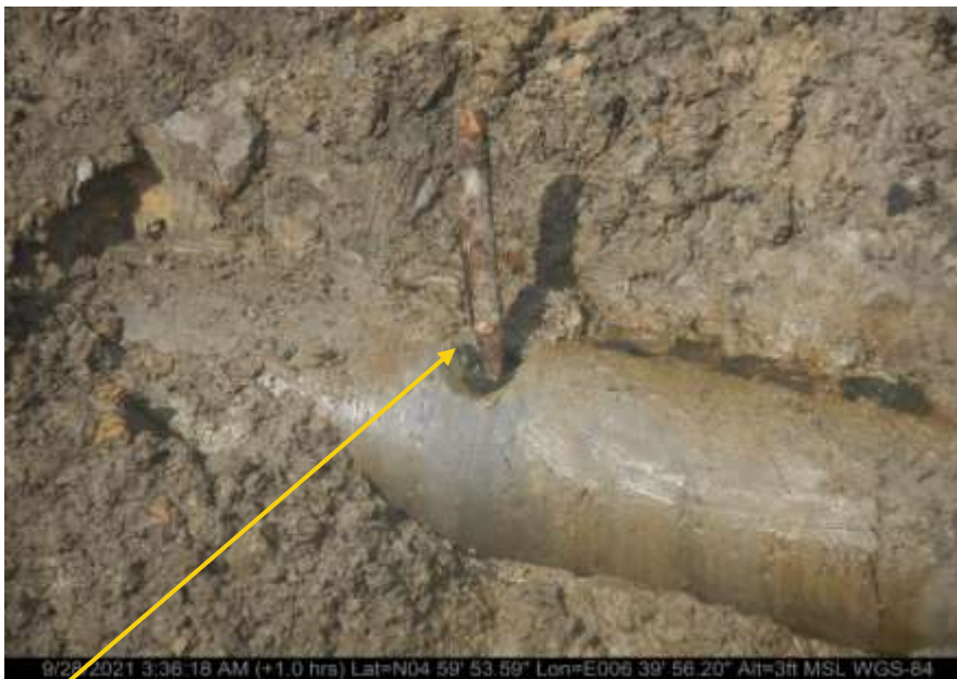
Close-up: Plugged round edge hole at 12 o'clock position on 14" Okordia Rumuekpe Pipeline at Ihuowo. Picture was taken during Joint Investigation of 28 th September 2021.
