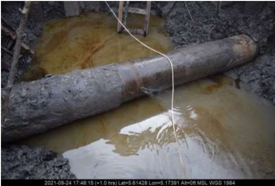
Overview: Part of spill impact on 20" Trans Escravos Pipeline at Ugboegungun. Picture was taken during Joint Investigation of 24 th September 2021.
