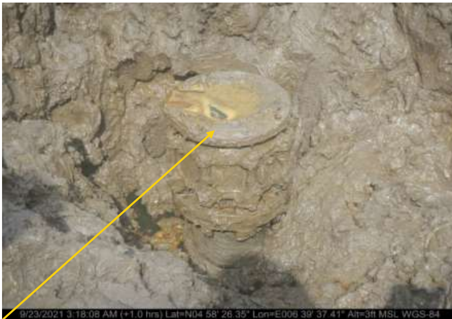
Close-up: 8inch ball valve installed at 12 o'clock position on 20" Kolocreek _Rumuekpe Trunkline at Okoma. Picture was taken during Joint Investigation of 23 rd September 2021.
