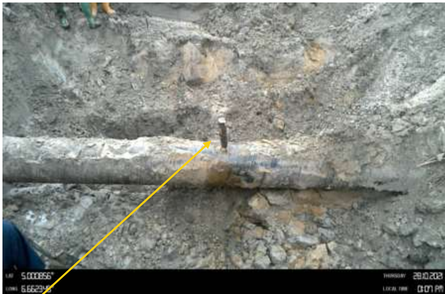
Close-up: Plugged 40mm smooth round edge hole at 12 o'clock position on 14" Okordia Rumuekpe Pipeline at Ihuowo. Picture was taken during Joint Investigation of 28 th October 2021.
