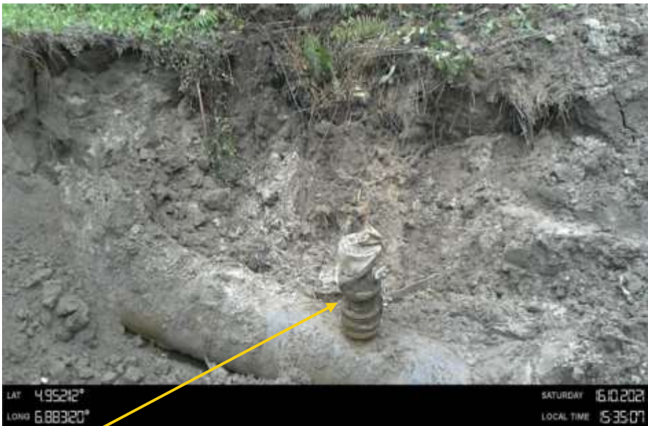
Close-up: 4inch Ball valve installed at 12 o'clock position on 20" Rumuekpe Nkpoku Pipeline at Adanta_Isiokpo. Picture was taken during Joint Investigation of 16 th October 2021.
