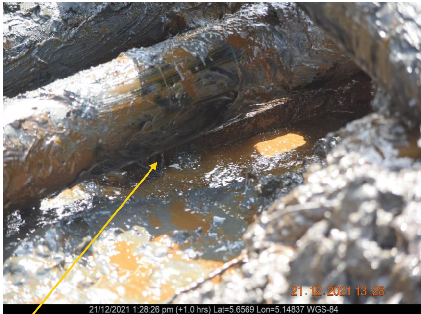
Close-up: Pin hole due to corrosion at 6 o'clock position on 4" Otumara Well 29S Flowline at Otumara. Picture was taken during Joint Investigation on 21 st December 2021.
