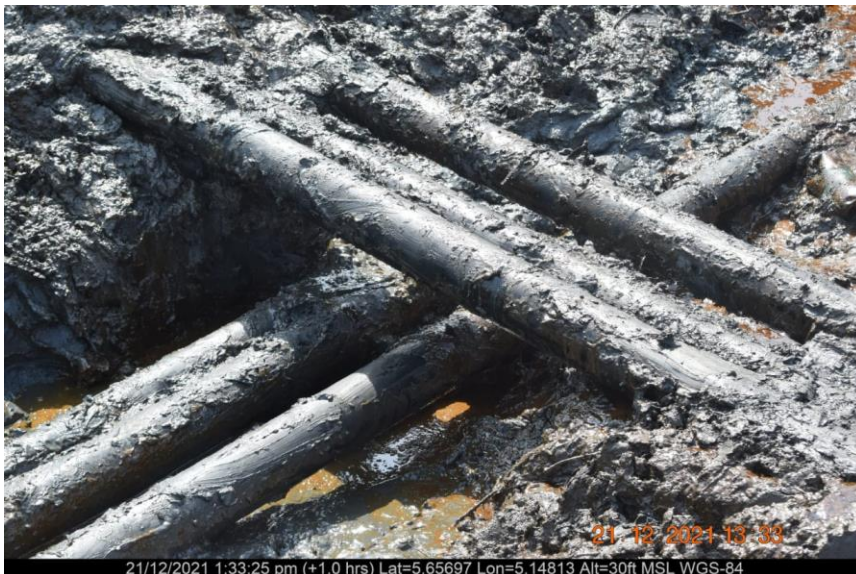
Overview: Part of spill impact on 4" Otumara Well 29S Flowline at Otumara. Picture was taken during Joint Investigation on 21 st December 2021.
