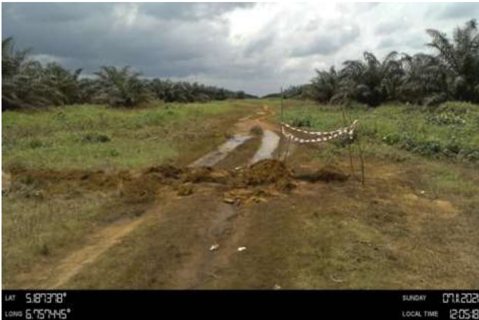
Overview: Part of spill impact on 18" Assa Rumuekpe Pipeline at Umudioga. Picture was taken during Joint Investigation of 7 th November 2021.
