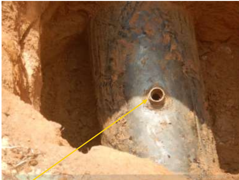
Close-up: Crude oil theft point installed at 12 o'clock position on 18" Assa Rumuekpe Pipeline at Umuodibe. Picture was taken during Joint Investigation of 24 th November 2021.
