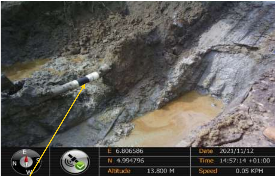
Close-up: Hack saw cut at 6 o'clock position with an arc distance of 90mm on 4" Obelle Ibaa Deliveryline at Ibaa. Picture was taken during Joint Investigation of 12 th November 2021.
