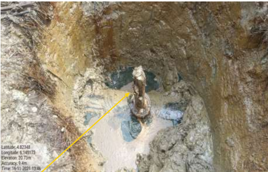
Close-up: Plugged 4inch flange installed at 12 o'clock position on 16" NunRiver - Kolokreek Pipeline at Aguobiri. Picture was taken during Joint Investigation of 16 th November 2021.
