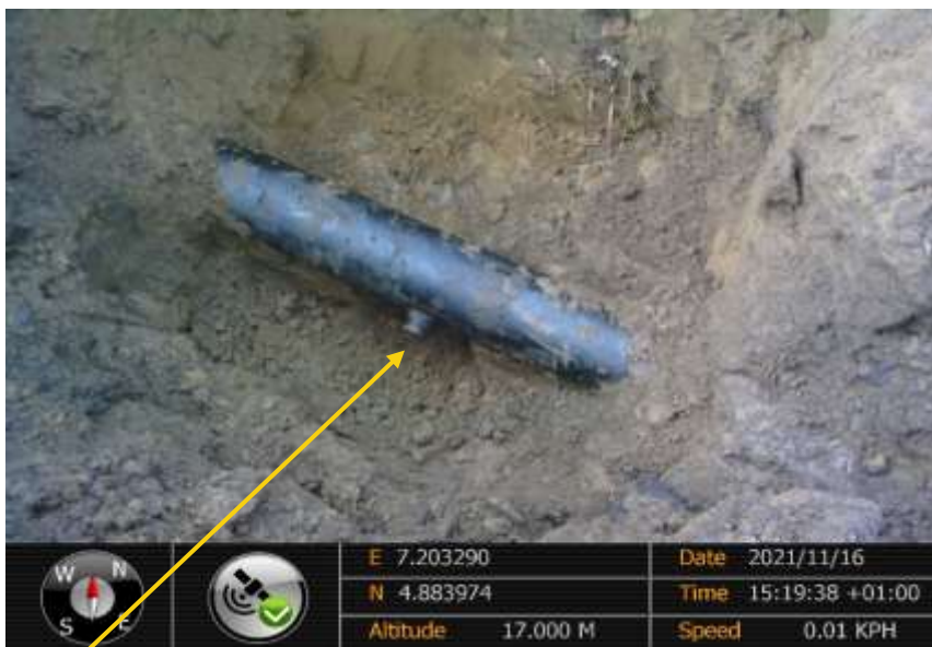
Close-up: 2inch nipple installed at 9 o'clock position on 8" Isimiri Deliveryline at Obiakpu. Picture was taken during Joint Investigation of 16 th November 2021.
