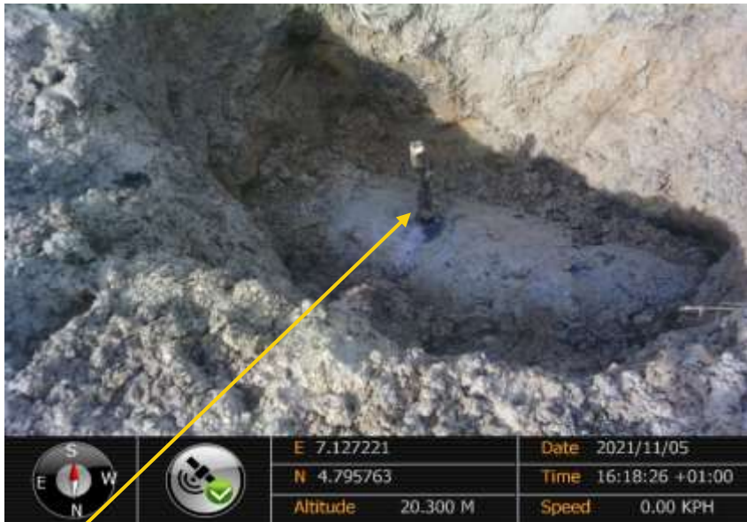
Close-up: Plugged 2inch nipple installed at 12 o'clock position on 28" Ogale_Bomu Pipeline at Agbonchia. Picture was taken during Joint Investigation of 5 th November 2021.
