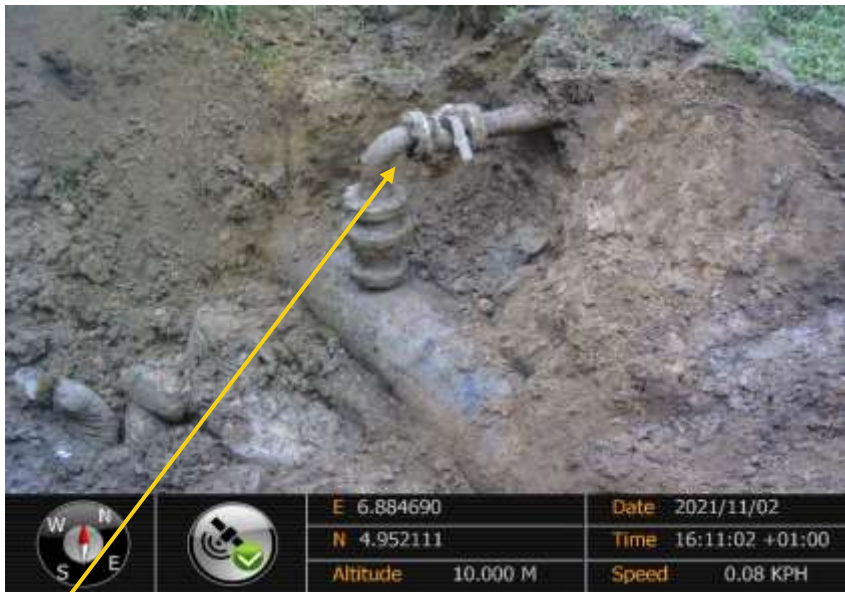
Close-up: 6''x 4'' ball valve installed at 12 o'clock position and fitted to 4'' extension pipe on 20'' Rumuekpe Nkpoku Pipeline at Adanta Isiokpo. Picture was taken during Joint Investigation of 2 nd November 2021.
