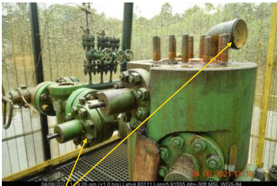
Close-up: Removed valves and survey cap on Seibuo Well 3 at Ogbainbiri. Picture was taken during Joint Investigation of 4 th June 2021.
