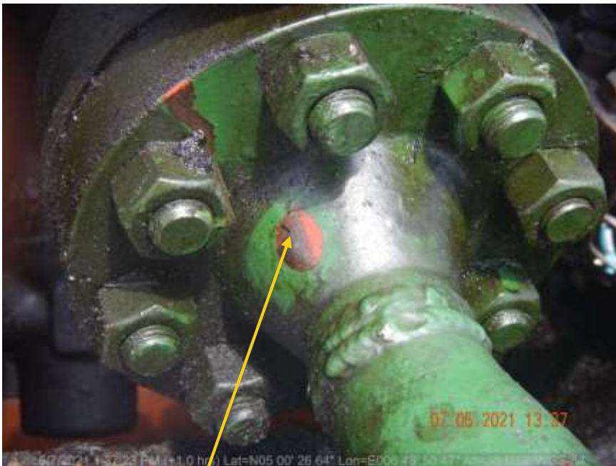
Close-up: Pinhole on 4inch Obele Well 3L flowline at Obele Picture was taken during Joint Investigation of 7 th May 2021.
