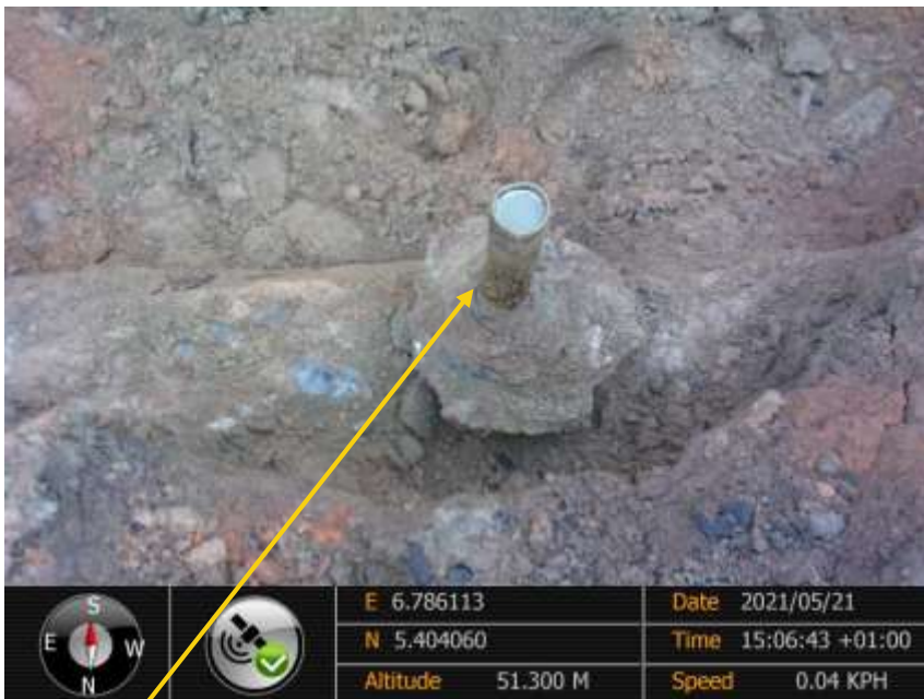
Close-up: 4inch ball valve installed at 12 o'clock position on 16inch Egbema Assa Pipeline at Obile. Picture was taken during Joint Investigation of 21 st May 2021.
